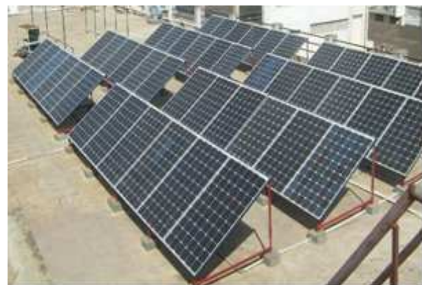
Fig. 3 The 10kWp roof-mounted PV system
